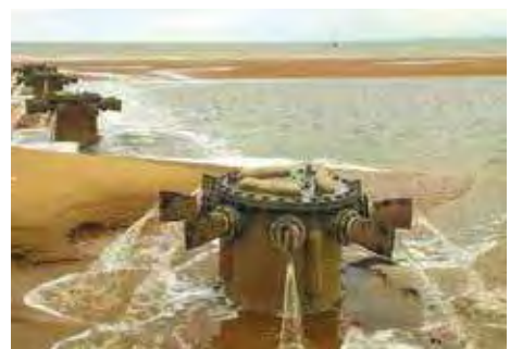
New diffusers installed as part of Morecambe Catchment Strategy – the ECC Options A and C scheme won Utility Project of the Year
