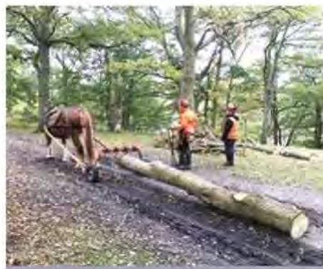
The main logs were locally sourced and dragged into position using a Suffolk Punch horse
