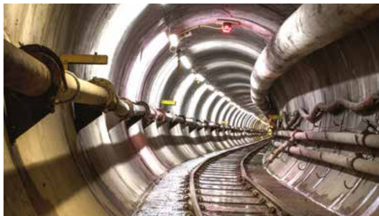
◀ The NEC-procured cable tunnel will supply the Battersea Power Station development, the Northern line extension and over 20,000 new homes
